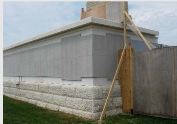
Newly engraved name panels sit above the three base courses of original stone, which were removed and redressed, before being relaid
